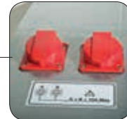
2 power sockets for one moulder and one divider
